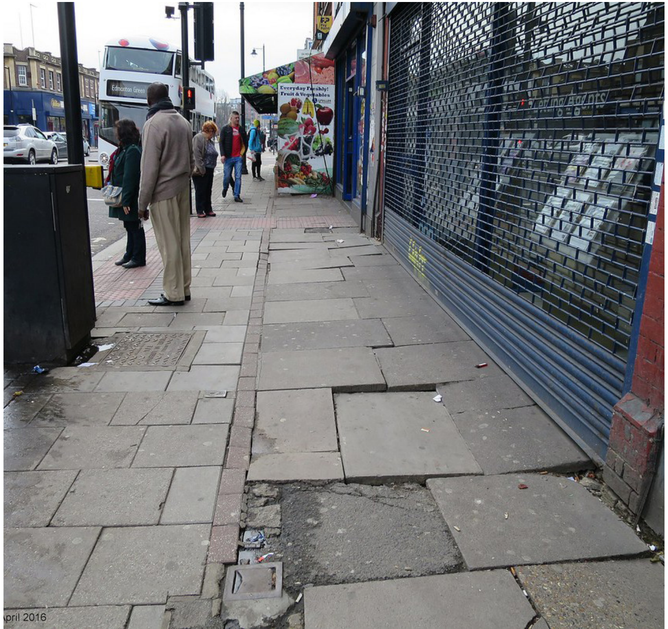
Damaged pavement slabs at 471 High Road - 2015
