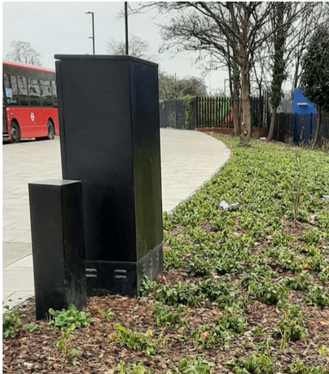
Utility cabinet – Tottenham Hale
